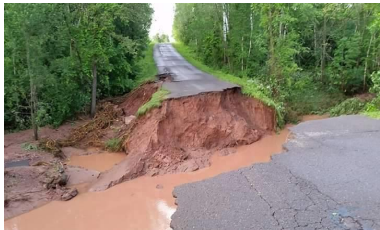
Figure 29. Failed culvert after severe storm on 7/11/16. Photo courtesy of the Bad River Band of Lake Superior Tribe of Chippewa Indians.
